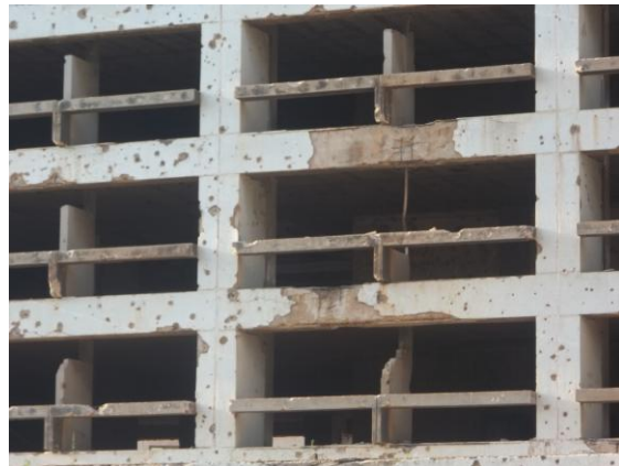
Figure 3b Holiday Inn on the Rouche, Beirut Lebanon 20 th /6 th /2011 Image taken by: Bilal Abou-Mosleh
